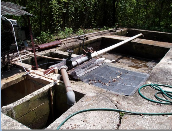
Prairie View package WWTF
