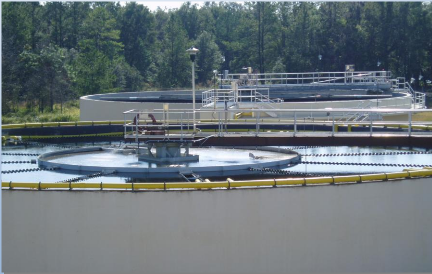
The clarifiers at the GRU Kanapaha facility
