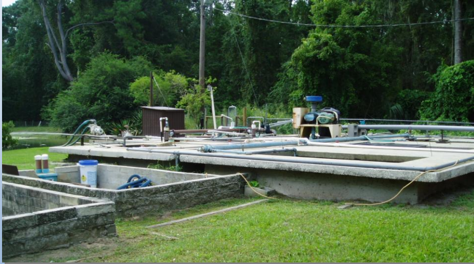
The Brittany Estates package WWTF
