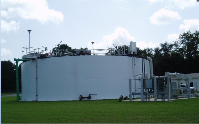
The City of High Springs WWTF
