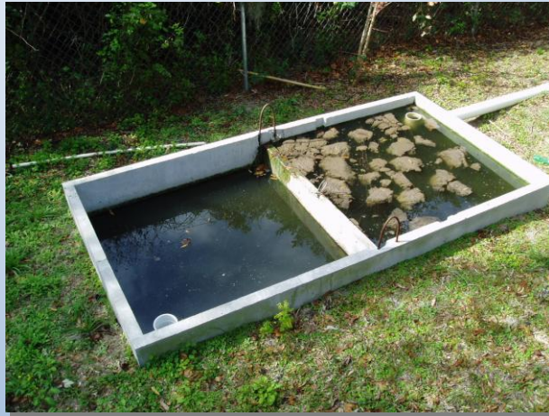
Solids in the chlorine contact chamber at the Archer Homes WWTF.
