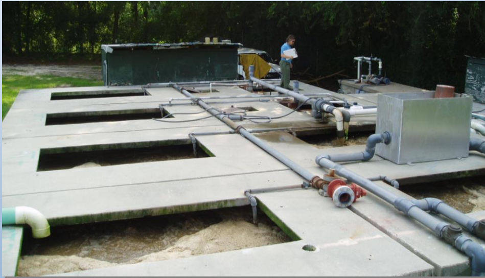
Aeration tanks in front of photo and inspector looking at one of the clarifiers in the rear of the package plant at the Arredondo Farms
