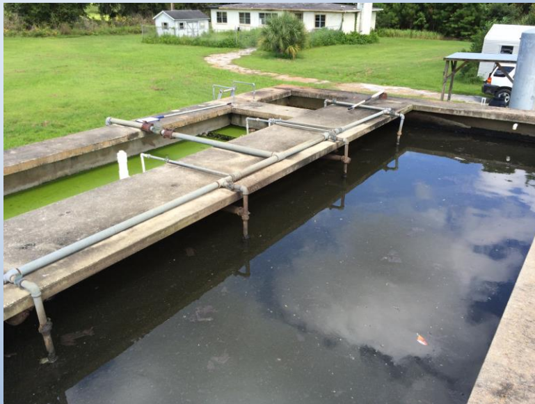
The Micanopy Inn aeration basin
