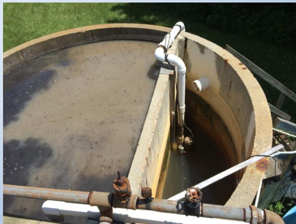
Camp Kulaqua clarifier and chlorine contact chamber
