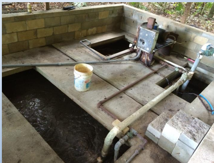
Camp McConnell YMCA aeration basin and clarifier
