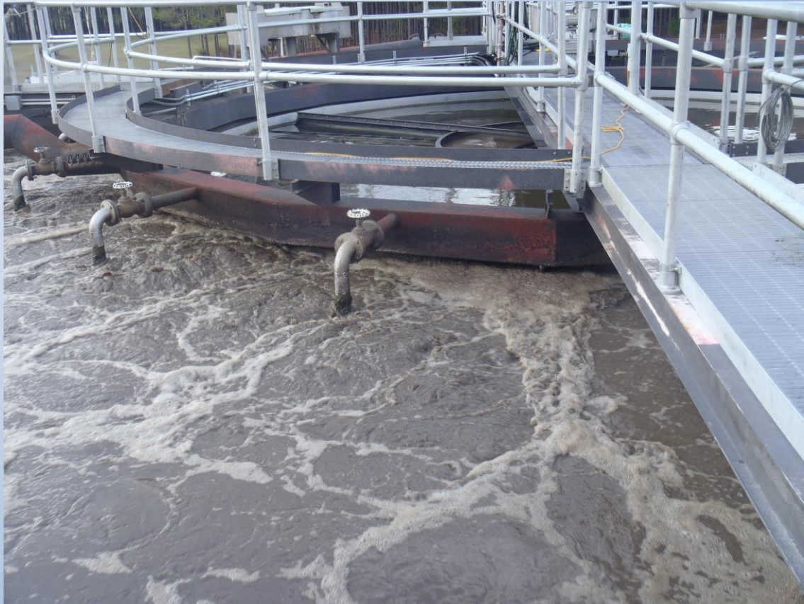
The City of High Springs aeration basin
