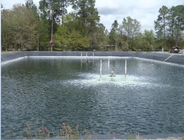
The Gainesville Raceway aeration treatment system
