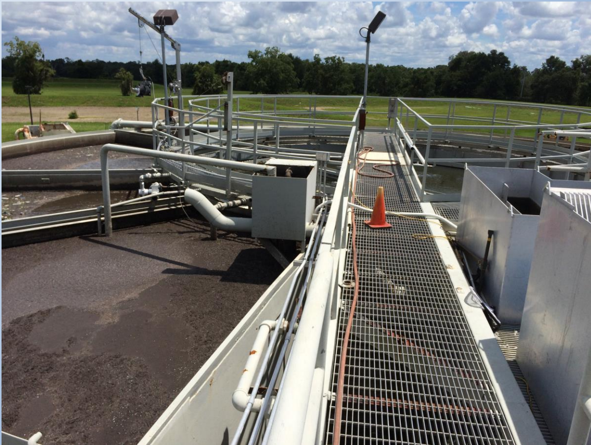
The City of Hawthorne Wastewater Treatment Facility
