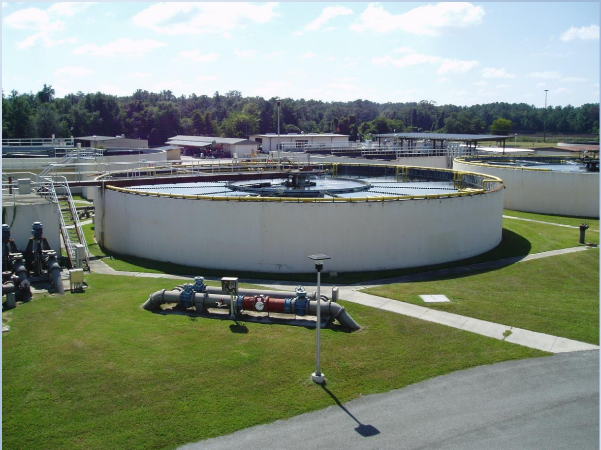
The clarifiers at the GRU Kanapaha facility
