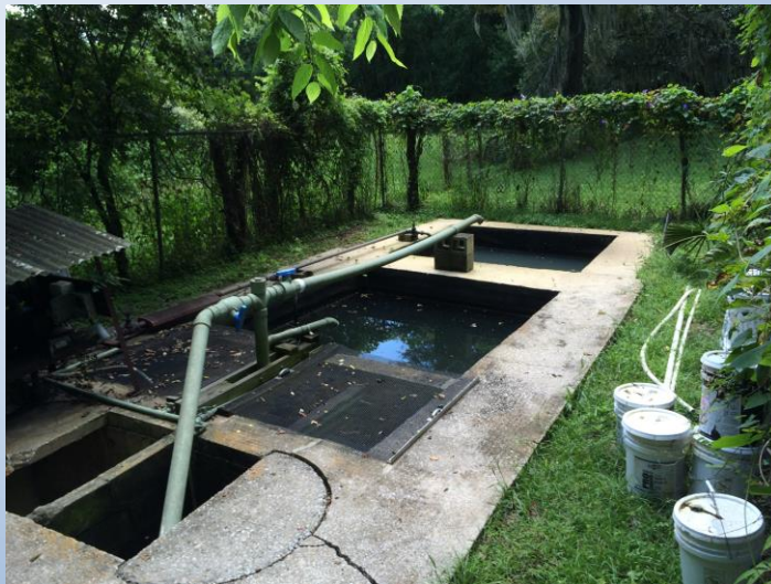
The Prairie View Apartments WWTF
