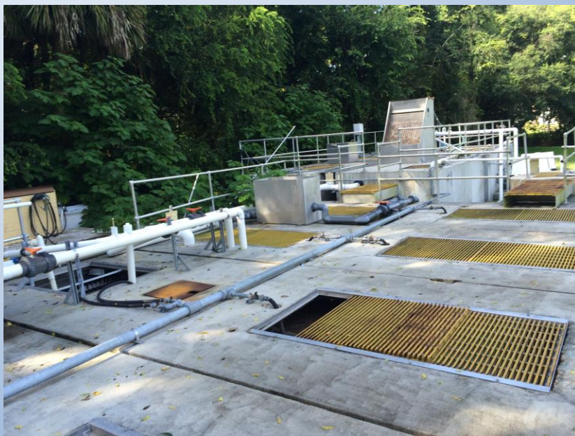
The Palms WWTf
