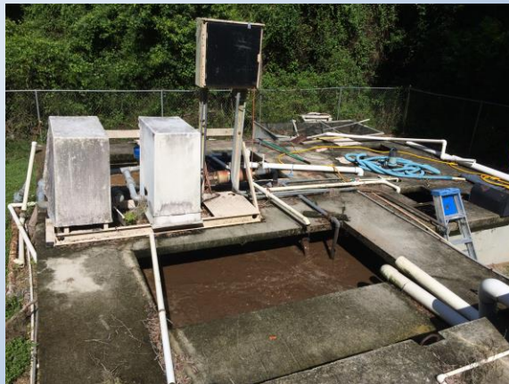
The Archer Homes WWTF
