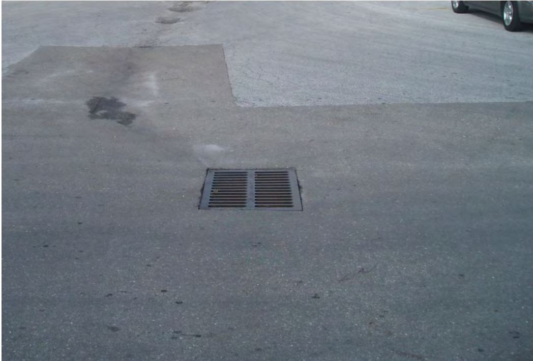
City of Gainesville Public Works Vehicle Inlet
