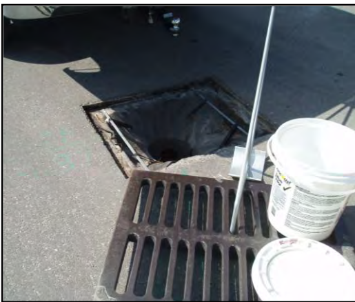
Stormwater inlet with inlet grate removed and Ultra-DrainGuard Oil and Sediment filter in place
