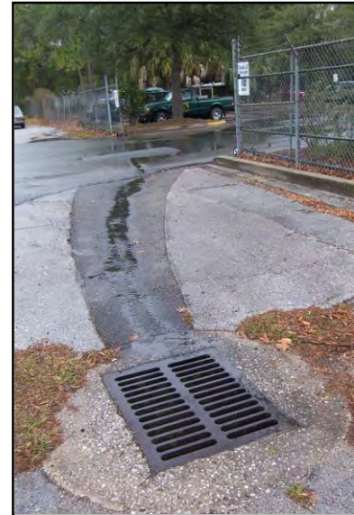
Stormwater inlet (FP North) collecting runoff from the Florida Pest Control & Chemical Company
