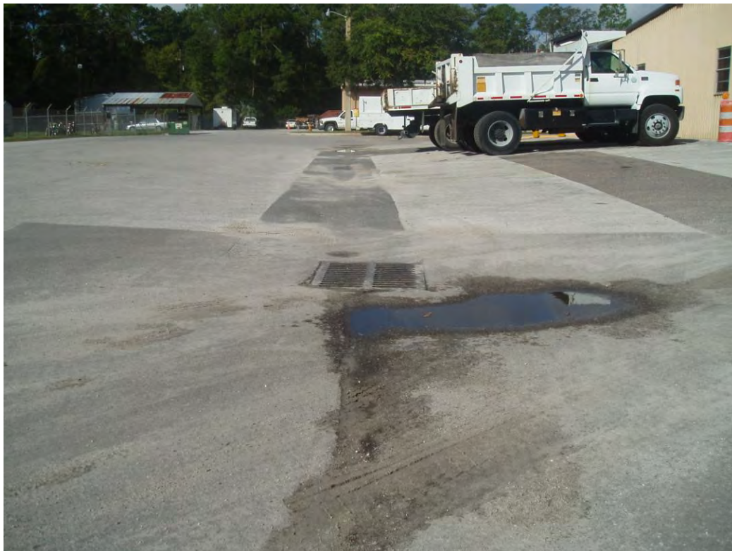
City of Gainesville Public Works Yard Inlet: note sediment
