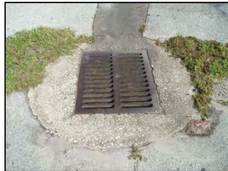
Drop stormwater inlet at Florida Pest Control & Chemical Company (FP North)
