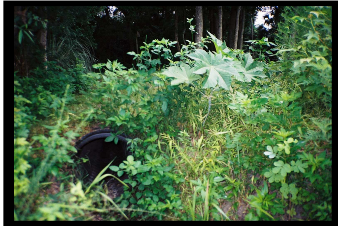
New Castor Bean at outfall of road drainage ditch. This is the result of a recent road paving project.
