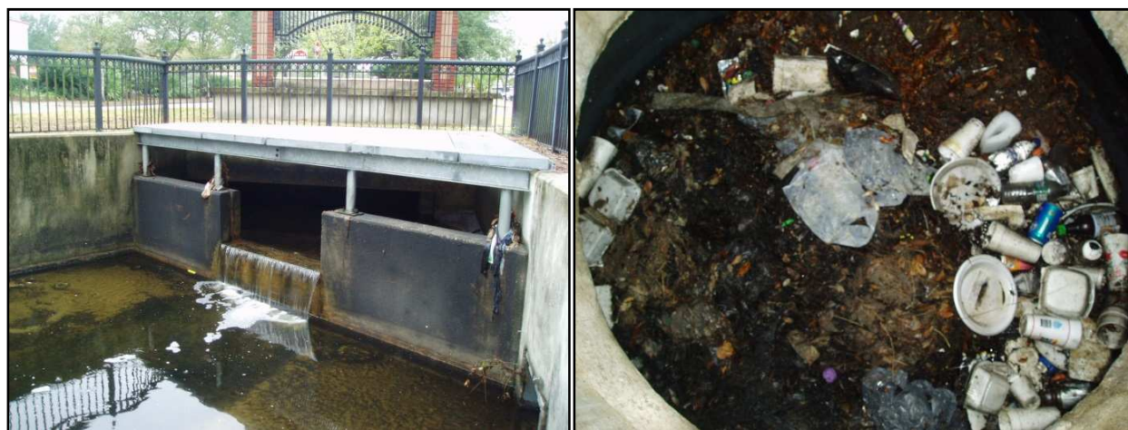
Figure A-2. Overflow weir on Sweetwater Branch at SWB10 (left) and SWB10BOX (right). December 12, 2012
